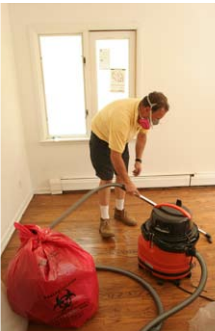
Final cleanup. After wrapping and bagging the floor plastic, vacuum and mop the floor. Use a disposable wet wipe to compare cleanliness to the cleaning verification card provided by the EPA.
