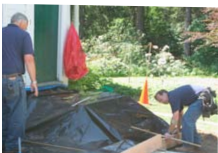
Contain paint chips at the edges. Turn the plastic edge up and support with lumber. Attach plastic to the house with furring strips, nails, and tape.
