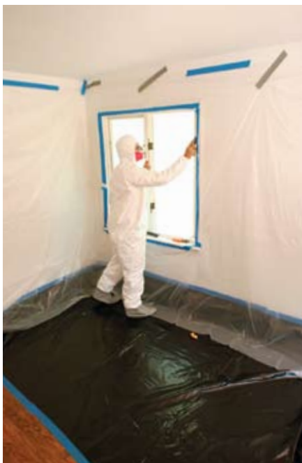
Set up a containment zone. Interior projects need a 6 ft. buffer zone that can catch dust and chips. Black plastic is a good choice on floors because chips and dust are more visible.
