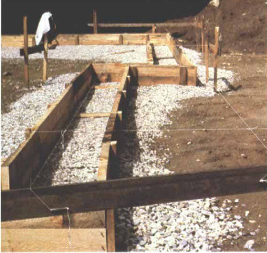
Forming and pouring the grade beam. At left, forms for the grade beam are being set up on top of the stone-filled trenches. The 2x10 form boards are held together by steel plumber's strapping and by 1x2 wood stretchers nailed across their tops. Below left, rebar has been placed between the forms, and tied off to spreaders. The transit mixer is discharging its load of concrete, which is being spread and leveled by the crew of Heartwood students.
