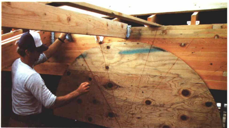
Once the curved header was installed, Phelps installed joist hangers radially every 12 in., left, to support the outside end of the dormer's 2x6 rafters. At the other end, above, he used strings and the cutout from the original plywood header template to lay out the locations of the joists' other ends.
