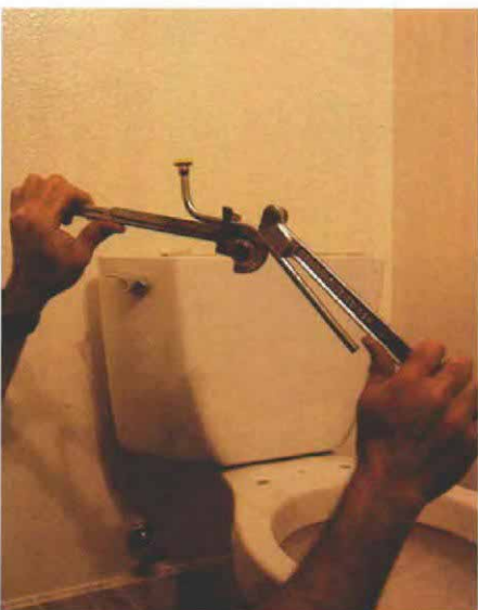
13. Skaates uses a tubing bender to shape the supply tube leading from the angle stop valve (lower left) to the toilet tank.
