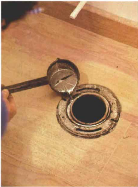
8. With the oakum in place, the gap between the drain and the flange is filled with lead.
