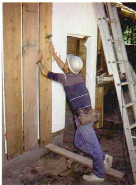
Hard-hat country. Working in tandem, one person on a ladder and another on the ground can install long boards easily with the help of a lever to hold the boards steady.
