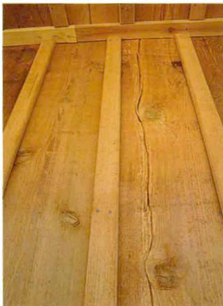
Wrong. Installed green with nails at the edges, this cedar 1x12 cracked down the middle as it dried out.
