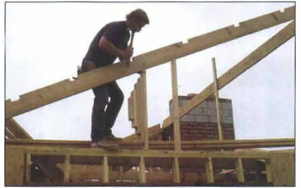
Installing the studs. Nail through the rafter into the studs to keep from putting a hump in the rafter.
