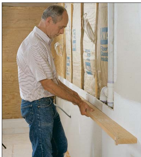
A straightedge can find a bowed stud. The straightedge alerts the author to this potential problem, which can be fixed before it interferes with a kitchen-cabinet installation.
