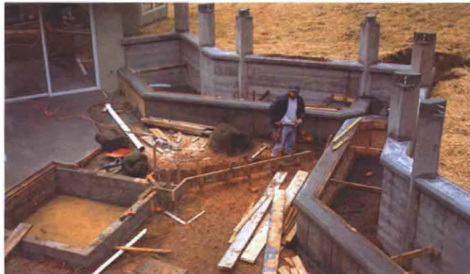
Not your average concrete pour. With the upper and lower pools cast, the job of linking them begins with the intricate formwork of the water channel. Drain lines in the lower pool and in the patio keep the water garden from overflowing.
