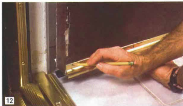
First the weatherstripping, then the door bottom. Weatherstripping is installed on the side jambs first. The drip cap on the door bottom then is scribed and notched to fit around the weatherstripping (11 and 12).
