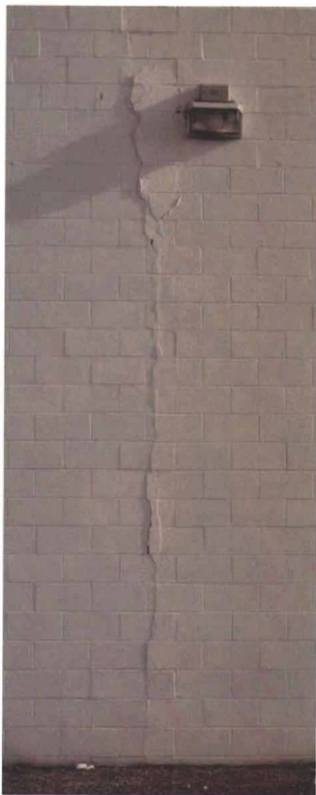
This wall made its own contraction joint. Quarter-inch contraction joints made of a high-grade elastomeric sealant allow a block wall to shrink as water dissipates from the grout, instead of cracking. This wall should have had these control joints every 15 ft to 20 ft.
