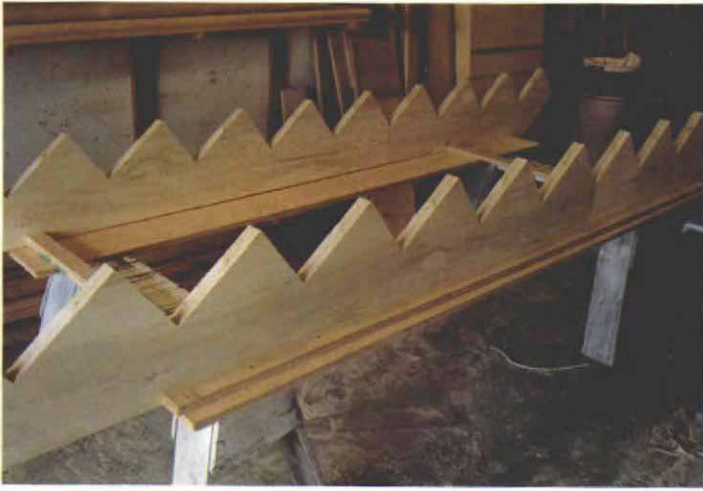
Assembly jig holds the stringers parallel and square. A simple jig made from strips of plywood holds the stringers at the proper width while the author is attaching treads and risers.
