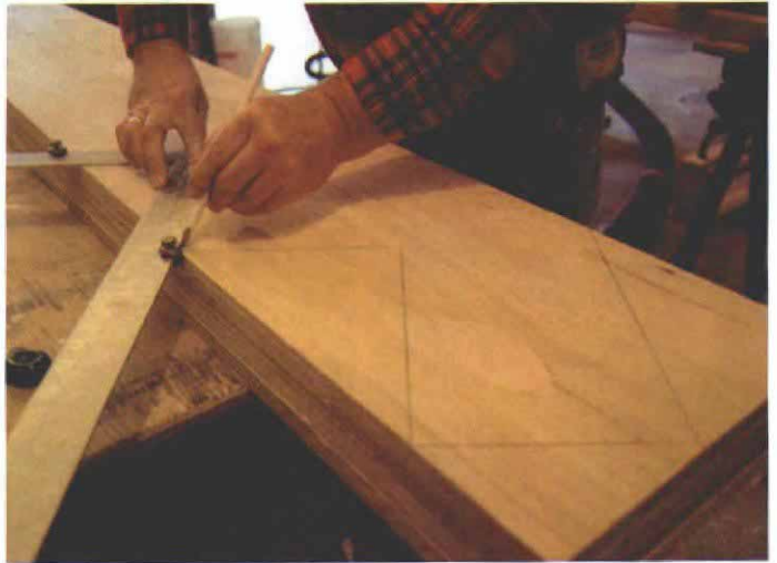
Each tread/riser layout is duplicated exactly. Stair gauges clamped to the edge of a framing square allow the layout to be repeated precisely for each step.
