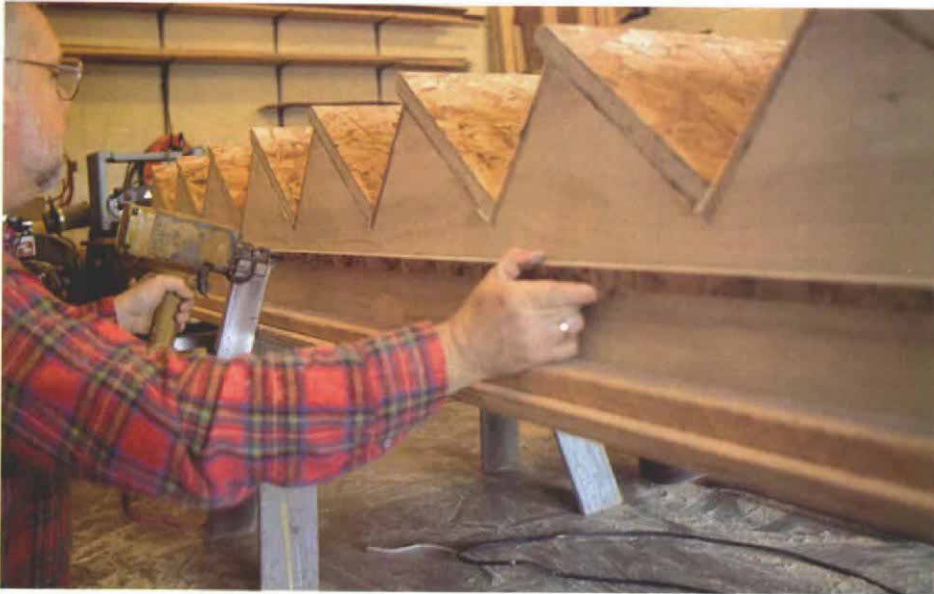
A spacer strip allows room for drywall. A 1-in. strip stapled to the stringer will keep the stringer away from the wall studs so that drywall can be slipped in behind the stringer after the stairs are installed.
