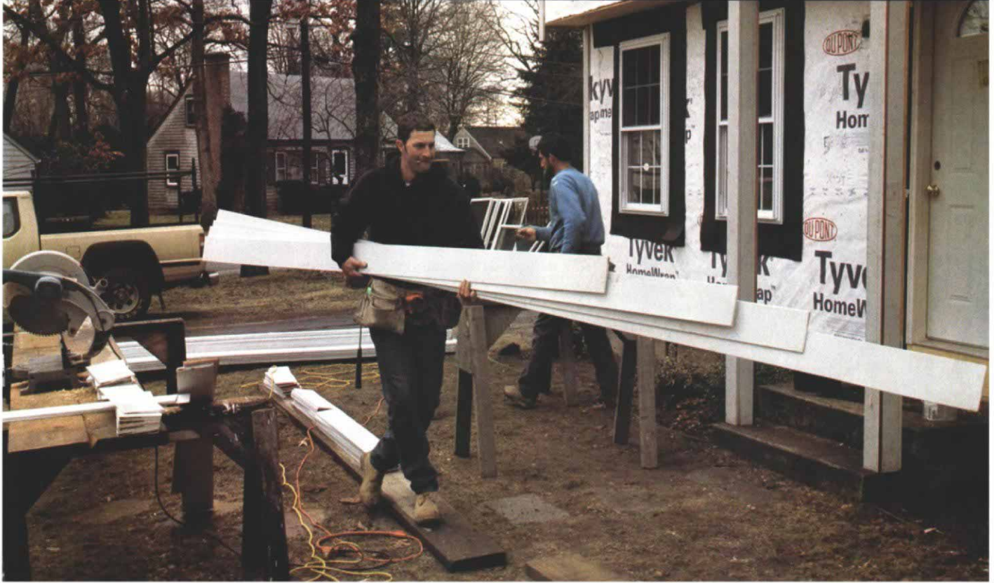
One carpenter nailed on corners and the water table, another cut the starter clapboards. He planned the cuts so that the joints are randomly staggered. Efficient crew members leapfrog each other, cutting or measuring ahead so that there is no downtime.
