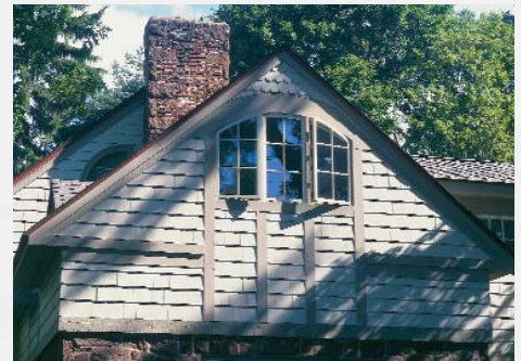
Divided elements create a unified appearance. The authors created visual interest by using vertical trim to emphasize the alignment of the upper and lower windows and to break up a large area of shingles.
