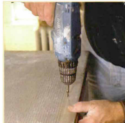
5. Screws hold the cement board down. Galvanized drywall screws 8 in. o. c. keep the cement board in place while the adhesive sets up.
