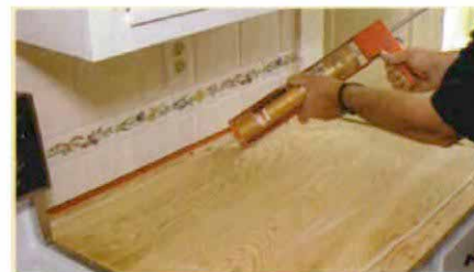
4. Bond the cement board to the counter. A bead of construction adhesive may be used to bond the cement board to the rough top.
