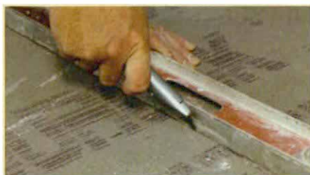
1. Score cement board with a knife. Tilesetter Tom Meehan uses a utility knife and a straightedge to score a piece of Durock cement board.
