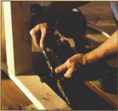
Air hose to the house. Instead of running the compressor off an extension cord, the authors make a run of hose by joining lengths of \frac{1}{2} -in. hose with threaded couplings (top photo) that have less air restriction than quick connects. In the house, a four-way splitter distributes air to the guns via easier-to-handle \frac{1}{4} -in. hoses (bottom photo).
