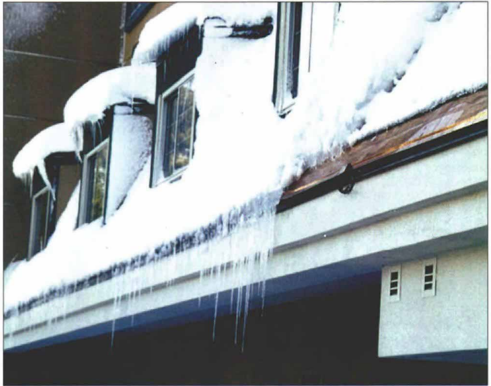
Heated eaves are one cure for ice dams. Warmed by electric cables, the copper eave in the foreground prevents ice dams that can cause leaks in the roof. The icicle-encrusted eaves in the background don't have heated metal eaves.
