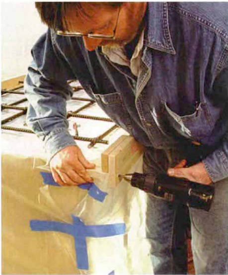
A gauge block sets counter thickness. The author uses a 2-in. wide block to locate the form edge. Because the screed will ride on the top of the forms, accuracy is important.
