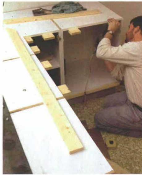
Braces are screwed to cabinet tops. To support the forms for the 2 3/4-in. overhang, Story uses deck screws to attach 1x bracing to the inside of the cabinets.
