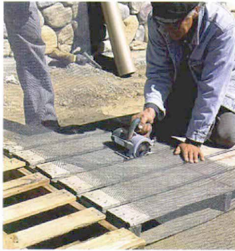
A saw keeps fingers away from sharp edges. Metal lath for the substrate can be cut with shears, but cutting with a diamond-blade saw is quicker and safer.
