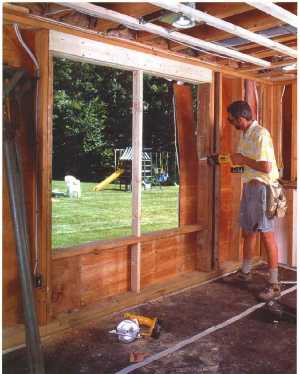
Let there be light. After the sheathing is nailed off around the perimeter of the opening, a reciprocating saw is used to cut back the sheathing, and the opening is ready for the new windows.
