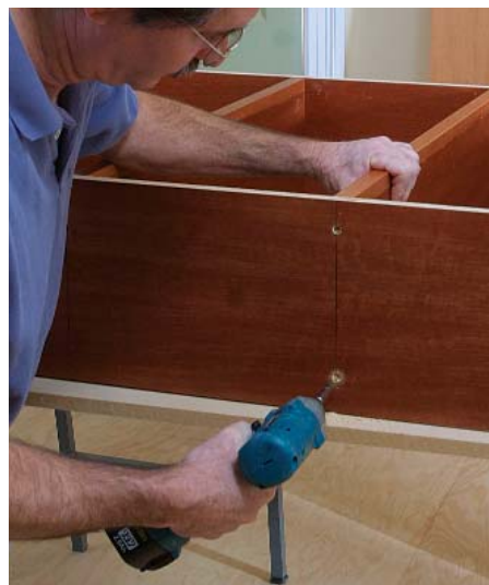
Pinpoint the screws. Once shelves are positioned, a line is drawn to center the fasteners (photo to left). Shelf is held against spacer while screws are driven through predrilled holes (photo right).
