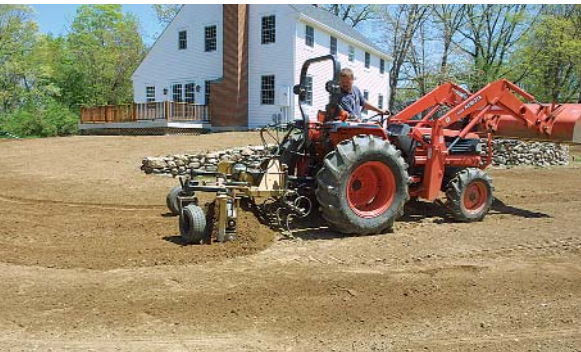
Machines to the rescue. On a larger site, a box rake speeds up grading. In a single pass, it can smooth and loosen soil while also separating debris.
