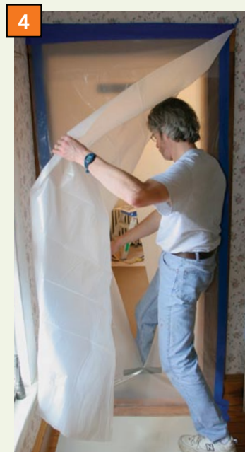
4 Trim the excess off the bottom of the second sheet of plastic where it meets the floor, and the homemade airlock is complete.
