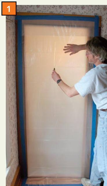
1 After taping all sides of the plastic, cut a slit down the middle, stopping a few inches short of the top and bottom.
