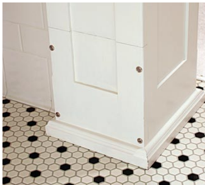
Don't forget the cleanout. Held in place by screws nesting in trim washers, a removable panel at the column base leads to the soil-stack cleanout.
