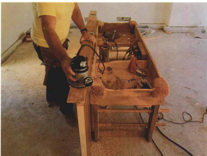
The same template used to rout the gains in the jambs is used to rout the gains in the edge of the door. The end of the template is flush with the end of the door. Note the template's round-head screw: it ensures 1/8-in. clearance between the door and the head jamb.
