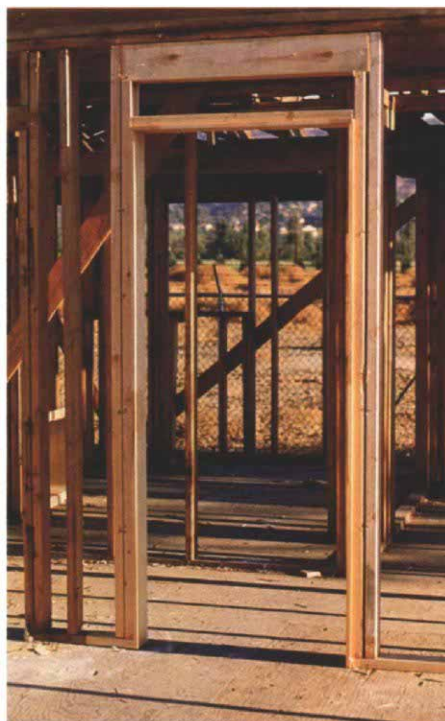
A clipped-trimmer door jamb stands in the foreground of southern California's Local 409 instructional framing project. Note how the header is just below the top plate, eliminating the need for cripples. The trimmers have been plumbed, straightened and clipped to the king studs, and the jamb has been affixed to the trimmers without shims. The portion of the sole plate that used to be between the trimmers has been removed and installed as drywall backing above the head jamb.
