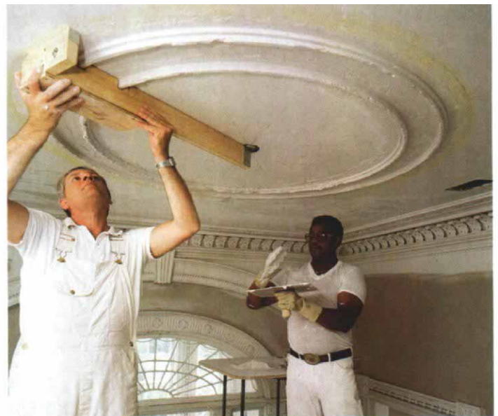
Assistant Richard Taylor trowels on a mixture of lime putty and plaster ahead of the template. It takes many passes with the template and some stuffing—swabbing plaster on rubber-gloved fingers—to eliminate voids.
