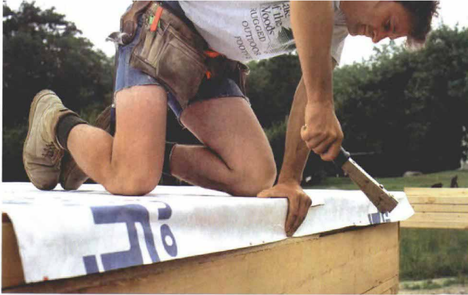
Tying up the loose end. At one end of the wall, the wrap is folded over the corner stud and stapled. After this wall is raised, sheathing from the adjoining wall will be nailed over the corner, holding the wrap in place.
