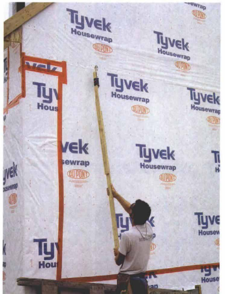
Extending your reach. For sections of housewrap that are hard to reach, such as between-floor seams, a hammer-stapler is taped to a furring strip to make fastening much easier.
