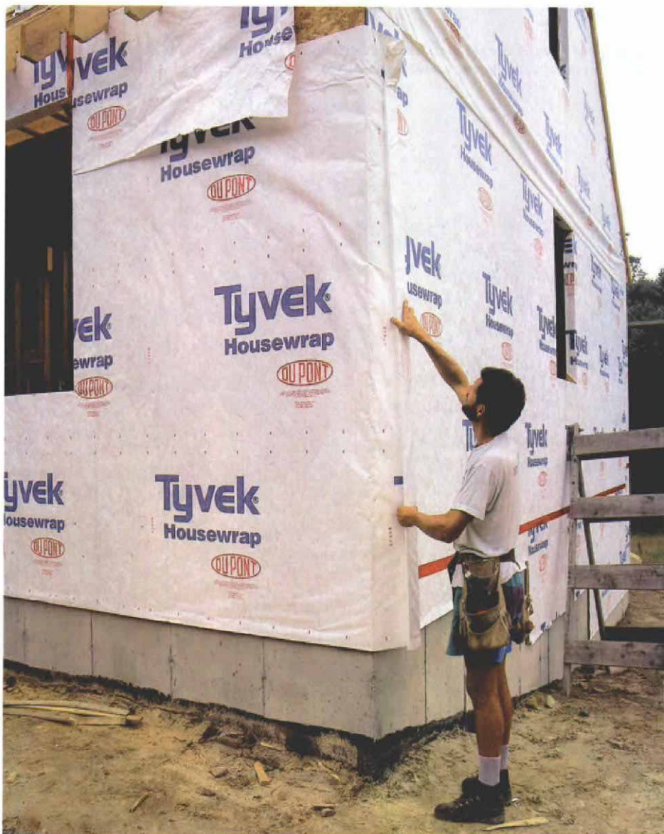
Corners are the last to be wrapped. On the opposite end of the wall, housewrap that earlier had been rolled up on a furring strip is unrolled and fastened in place, which happens after the framing is tied together with the final pieces of sheathing.
