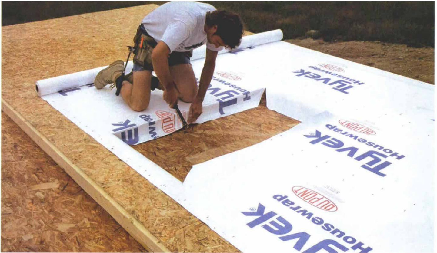
Housewrap is cut to fit framed window openings. Instead of the standard X-cut for a window opening, the housewrap is cut to cover just the framing to eliminate large flaps that are likely to tear in the wind.
