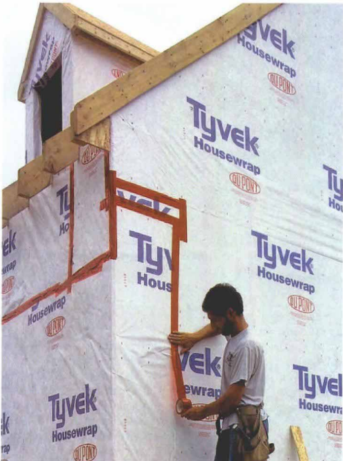
Sealing the corners. The authors try to tape the corner seams of the housewrap as soon as possible after the wrap is installed to prevent any possible wind damage.
