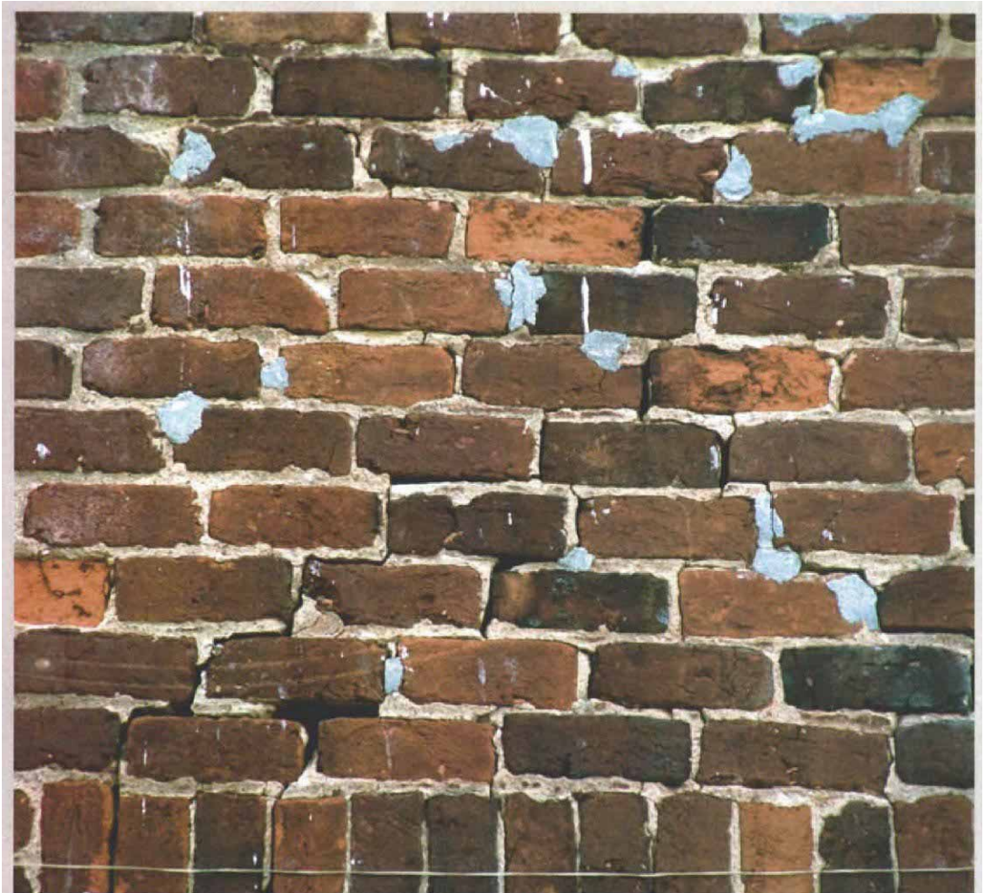
Look for continuous or zigzag cracks in masonry walls. Although small cracks are to be expected, the long, continuous cracks in this old brick wall suggest that the footing and foundation have settled.
