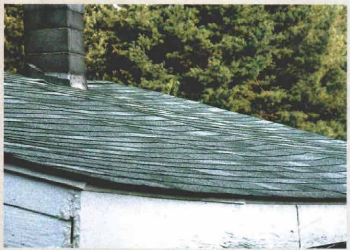
A roof should be straight. A wavy roof deck can indicate that the underlying sheathing is too thin or starting to rot or delaminate. A sagging ridge may mean the same thing.
