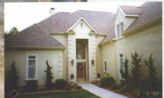
Be wary with stucco finishes. It pays to be careful when inspecting a house with a stucco exterior. From the outside, nothing seems wrong with this barrier-type synthetic-stucco exterior (inset). Inside the wall, it's a different story.
