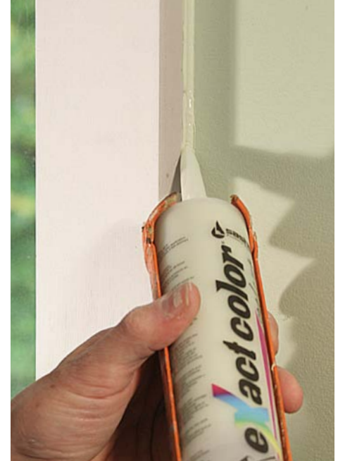
Caulk neatly. After allowing 30 minutes for the activator to thicken the caulk to a normal consistency, fill the joint.
