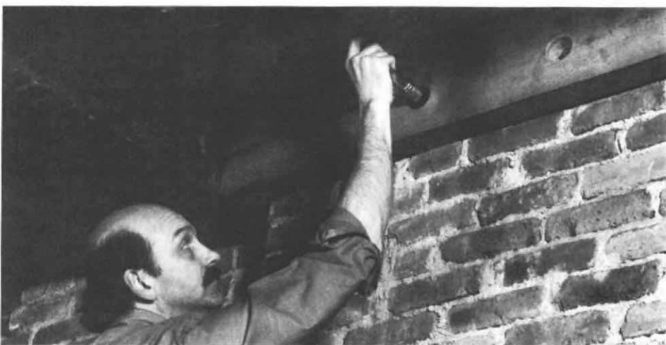
A plywood sheet, top, temporarily replaces the third-floor hearthstone. The face course below has been relaid using the original bricks and repointed to match the style of the original chimney. Above, bolts sunk in the reconstructed face course just below the third floor secure a new chimney girt, to the wall. This will support a new section of floor that replaces the third-floor hearthstone.
