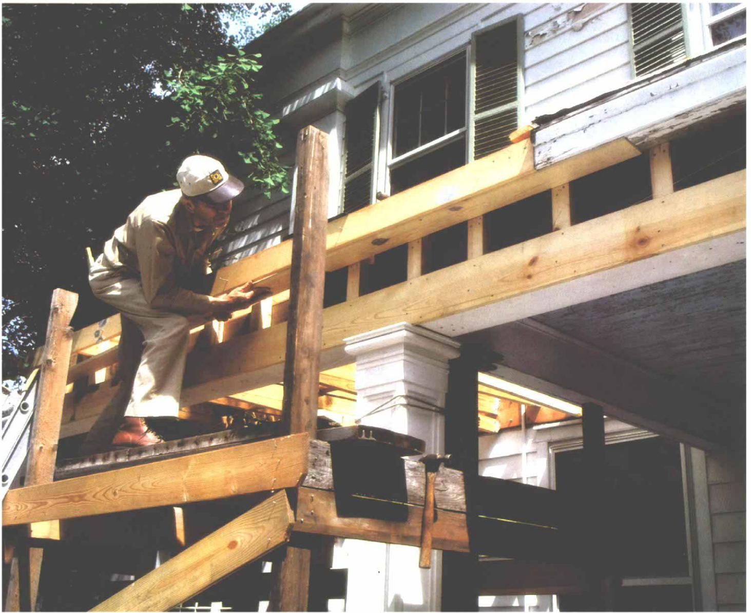
Test-fitting the soffit in the new roof. Joints between old and new soffit, fascia and frieze boards are staggered for lateral strength and to make the addition as inconspicuous as possible. One-by-three spacers build out the fascia to the full width of the column.
