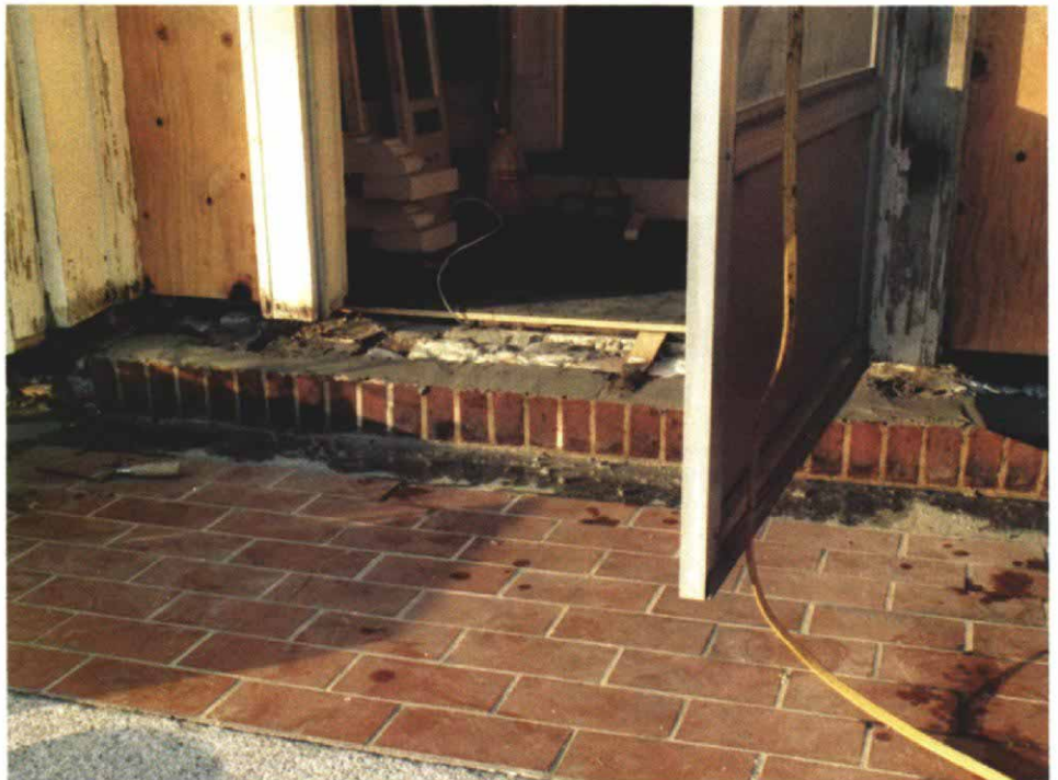
To start the job, Sewall removed the doorway's side lights and nailed plywood panels in place, with clearance beneath them to slide in the new sill. Then he removed the original sill, which had been resting on 1-in. strips of wood set in a bed of mortar.
