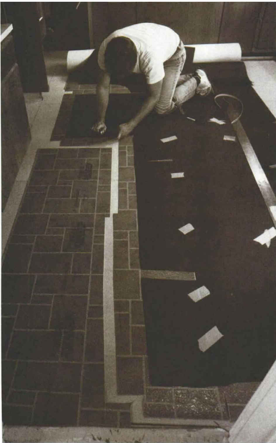
Two 3-ft. wide pieces of builder's felt are butted together and taped to make a pattern for the first drop in the kitchen shown in the drawing on the facing page. Here the finished pattern has been taped onto the flooring, and Shrode is trimming the material to fit. The corner cut-out at the bottom of the photo indicates that this will be a coved floor.
