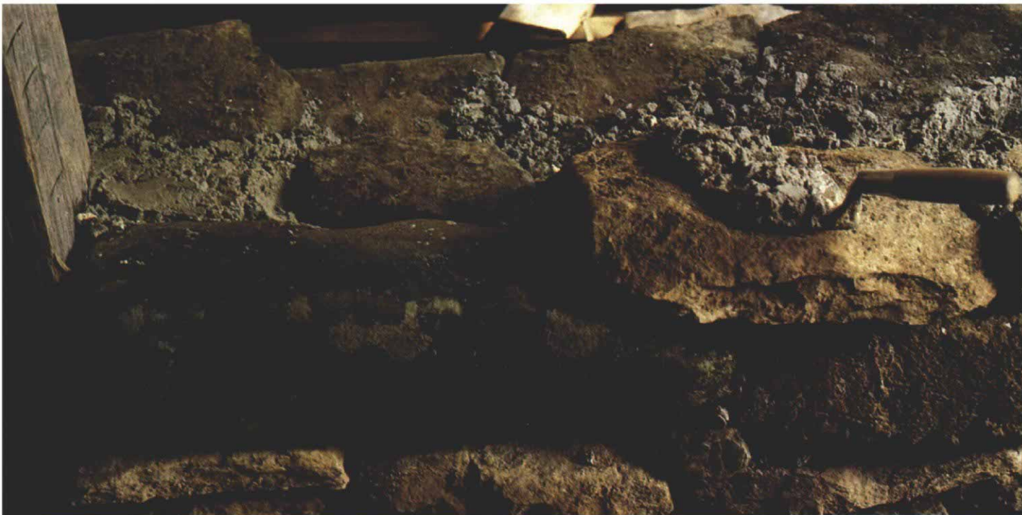
The heart of the wall. The ingredients are stones and a very dry, stiff mix of concrete. The stones are gravity fit with overlapping joints. Concrete and small stones are used to fill the voids between larger stones. As the wall is built, the concrete is kept back at least an inch from the face of the wall. This leaves enough space between stones for a thin, strong mix of pointing mortar.
