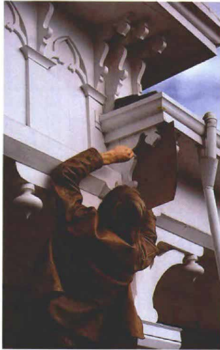
To produce a durable pattern for bandsawn Victorian brackets, Hap Tallman uses hardboard, and traces the shape directly from the original bracket. So far he's collected over 40 bracket designs.
