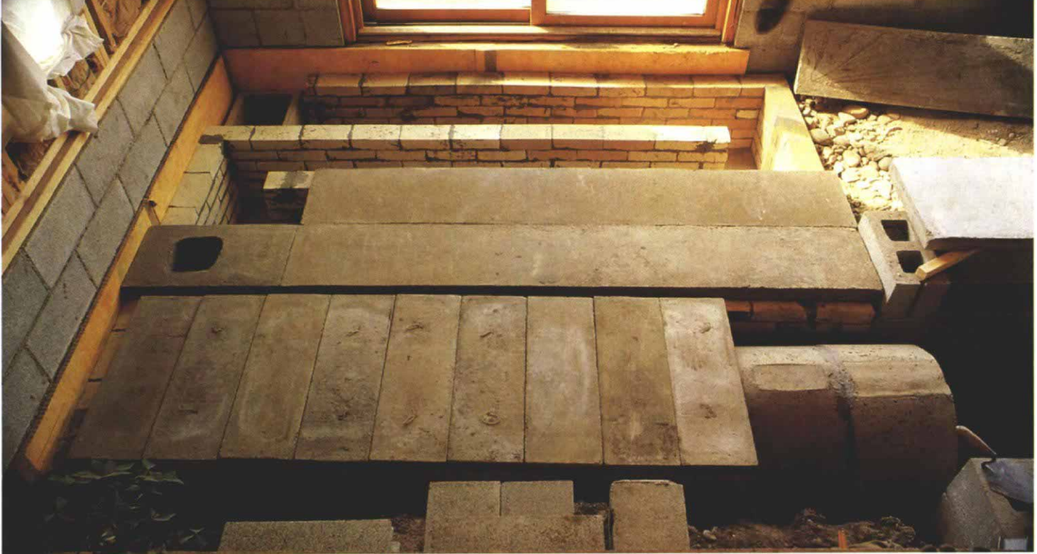
Like the firebox arches, the lids of the first three flue runs were also precast with refractory concrete. To allow for extra expansion and contraction due to the high temperatures, Marcus used nine separate sections to make the lid of the expansion chamber.
