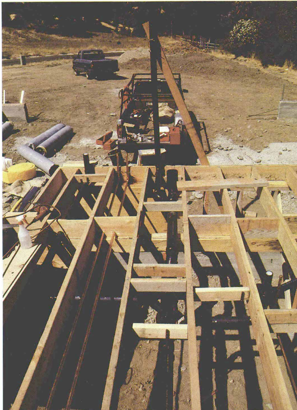
Under the floor. In the center of the photo, a 3-in. soil line leads to a 4x3 closet ell. A few feet in front of the ell, a 3x2 sanitary tee turned at a 45° angle leads to a vent for the water closet. At the plate line, the vent is extended upward with a 10-ft. mast for a water test. To its left, a branch line goes to a stub for a lavatory and an upstairs laundry. In the lower right, a stub protrudes for a bathtub. The drain line in the center is secured with a plastic hanger.
