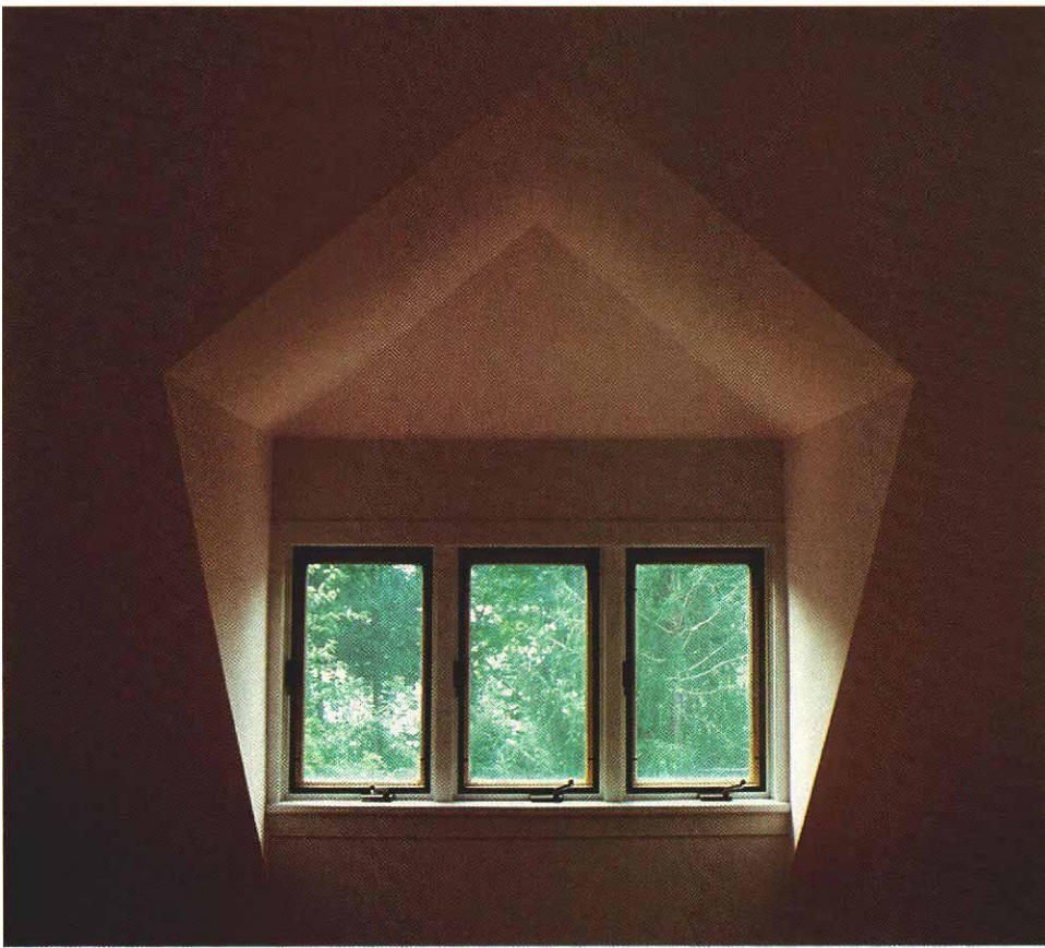
Although this dormer has a hip roof, it was framed with the valley-rafter method and illustrates the clean, geometric ceiling lines that make the complexity of this framing worthwhile.
