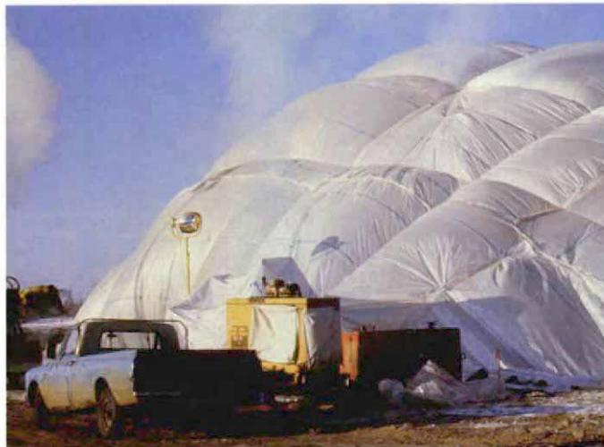
Enclosures can be made of polyethylene sheeting and inflated with heaters and blowers to cover everything from slabs to entire houses.
