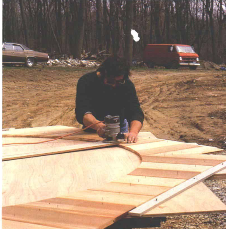
With the cedar siding tacked in place on the trammel jig, Goodale pivots the swing arm and neatly trims the boards for a perfect fit against the arch-top window.
