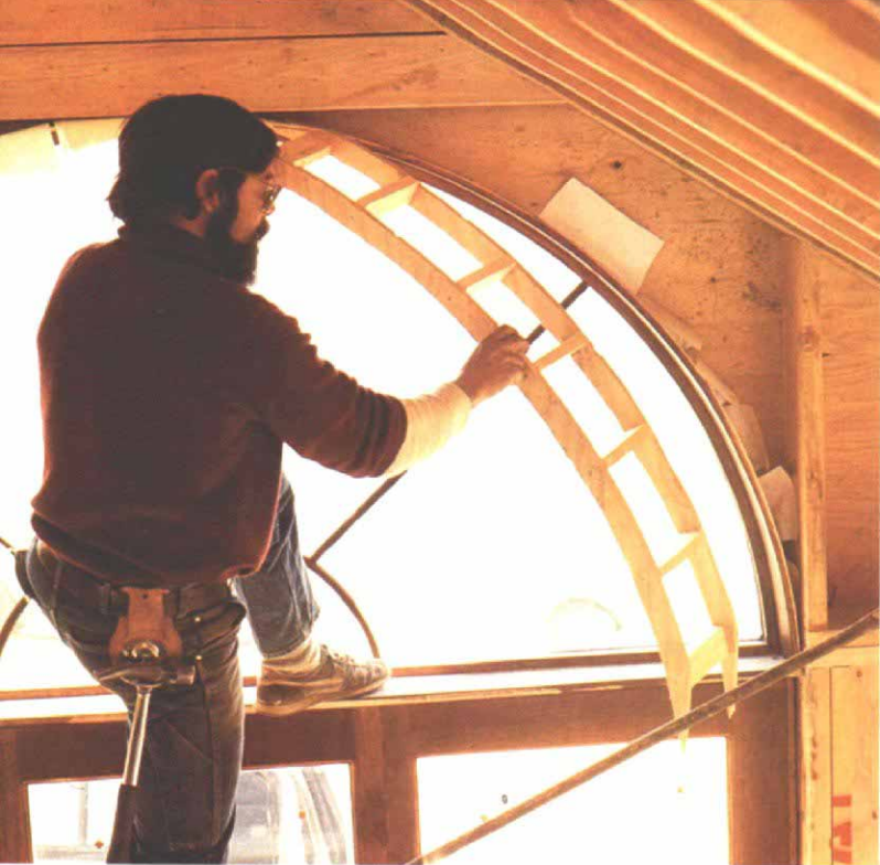
To provide nailing for sheathing, drywall and trim around arch tops, Goodale installs curved ladders made of plywood sides with blocks nailed between them.
