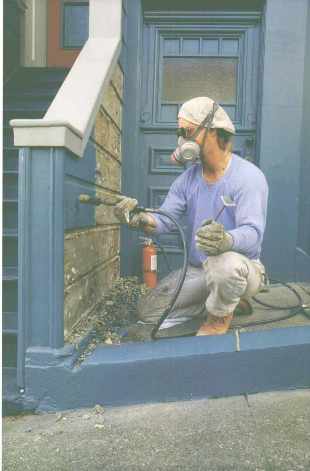
A torcher at work. The quickest way to remove failing paint from wood siding is to scrape it off after softening the paint with a propane torch. When doing this work, it's imperative to wear safety gear and to have fire-fighting equipment nearby.
