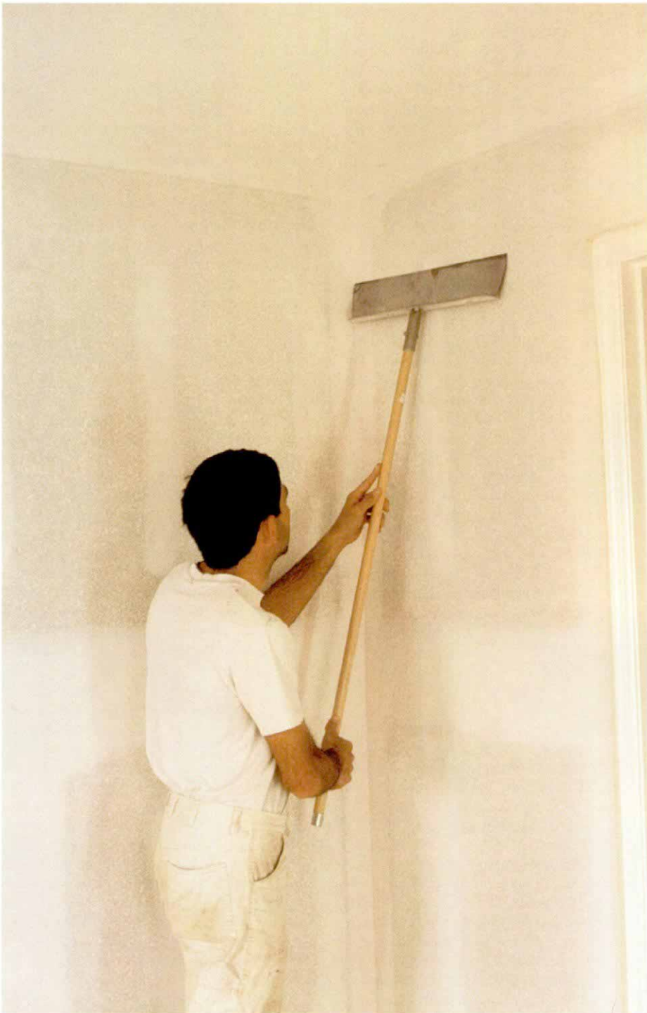
Last-minute touch-up. Textures can mask slight surface irregularities, but walls that have a sprayed-on "orange-peel" texture often have some large clumps that need to be taken off before painting begins. The author uses a drywall scraper to remove them.
