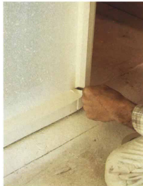
The tip of a pocket knife is a handy tool for sticking down the working edge of a run of masking tape. The intersection of baseboard and casing is vulnerable to leaks and needs to be thoroughly sealed. Note how the tape overhangs the baseboard, acting as an umbrella to shield it from roller spatter.
