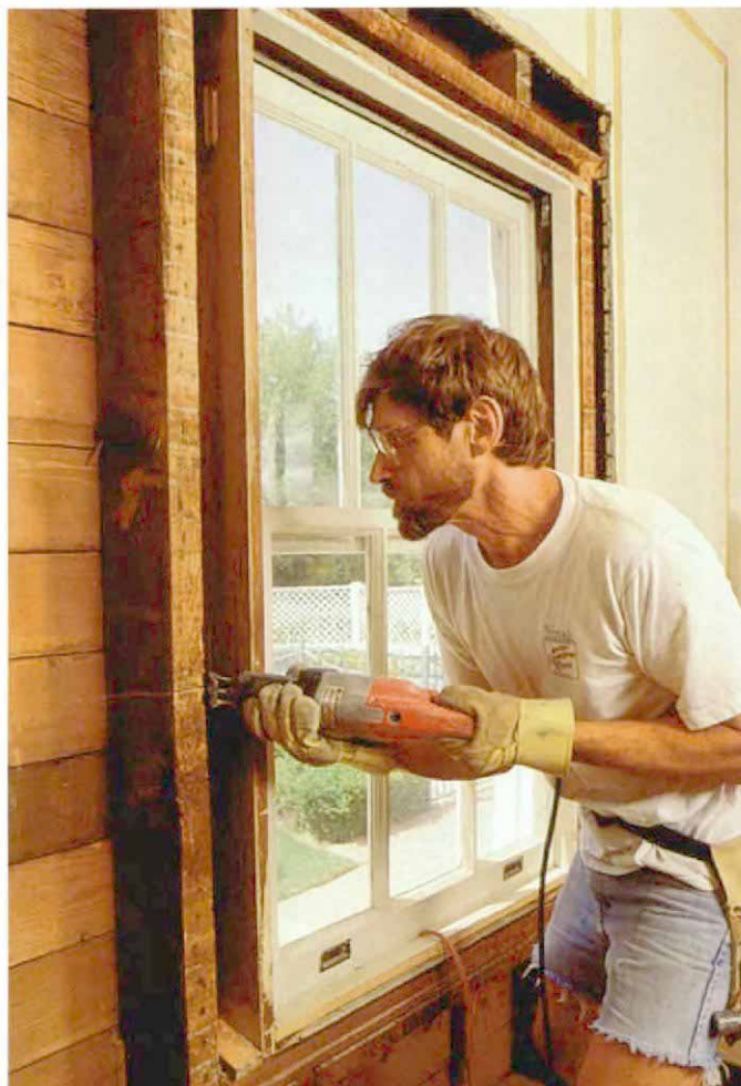
Out with the old. A reciprocating saw makes short work of old plaster, studs and the nails that hold them together.
