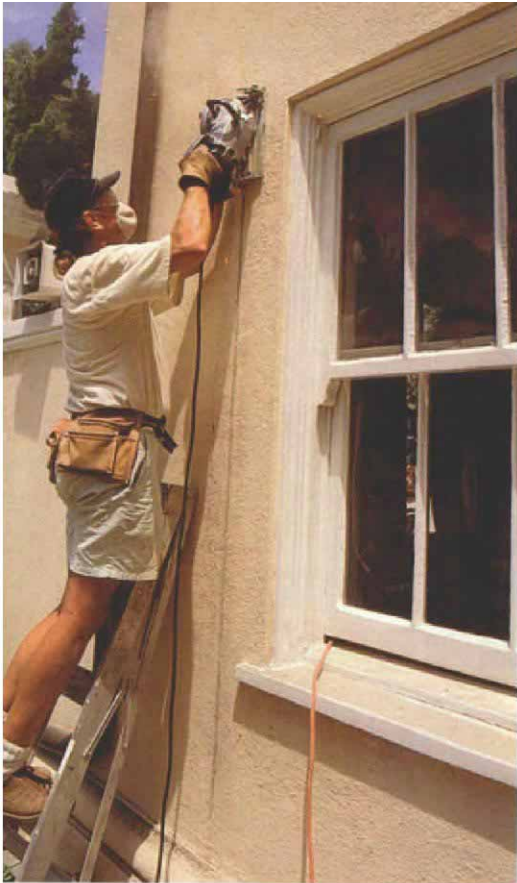
Using a Carborundum masonry blade ensures a straight, clean cut in a stucco wall.
