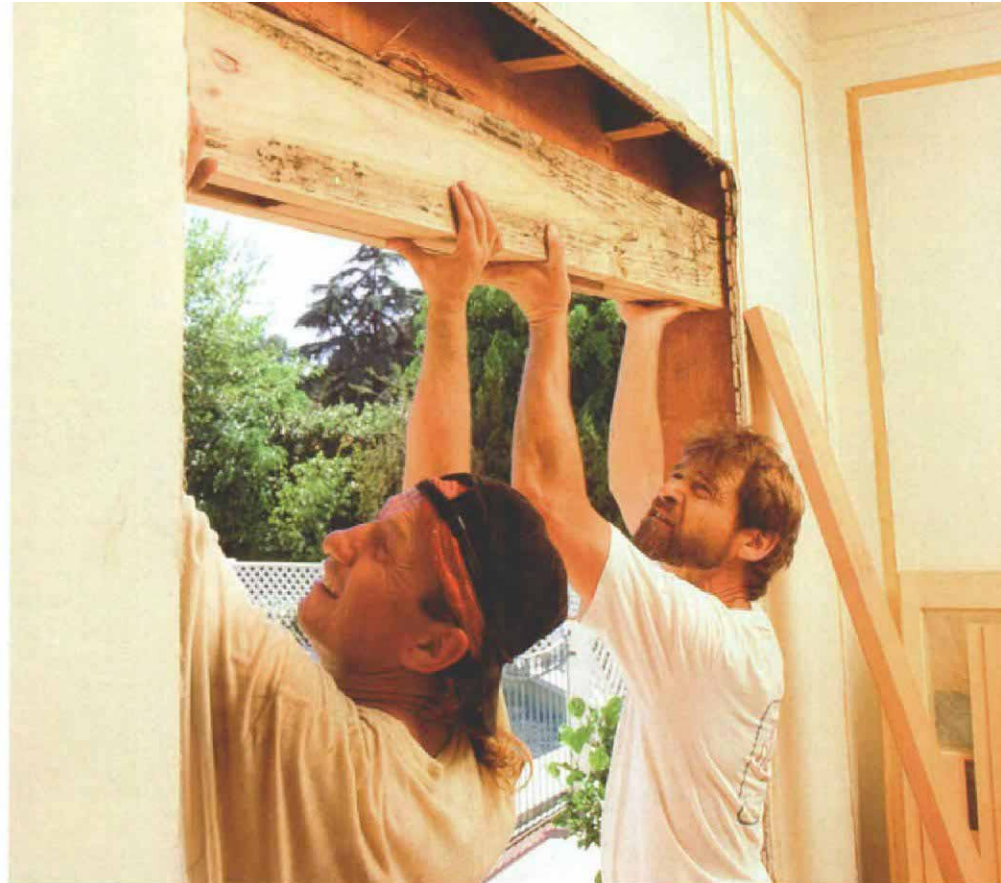
The new header is inserted into its cavity in the old wall. Note how the cripple studs over the window have been cut in a horizontal line so that they can bear equally on the header.
