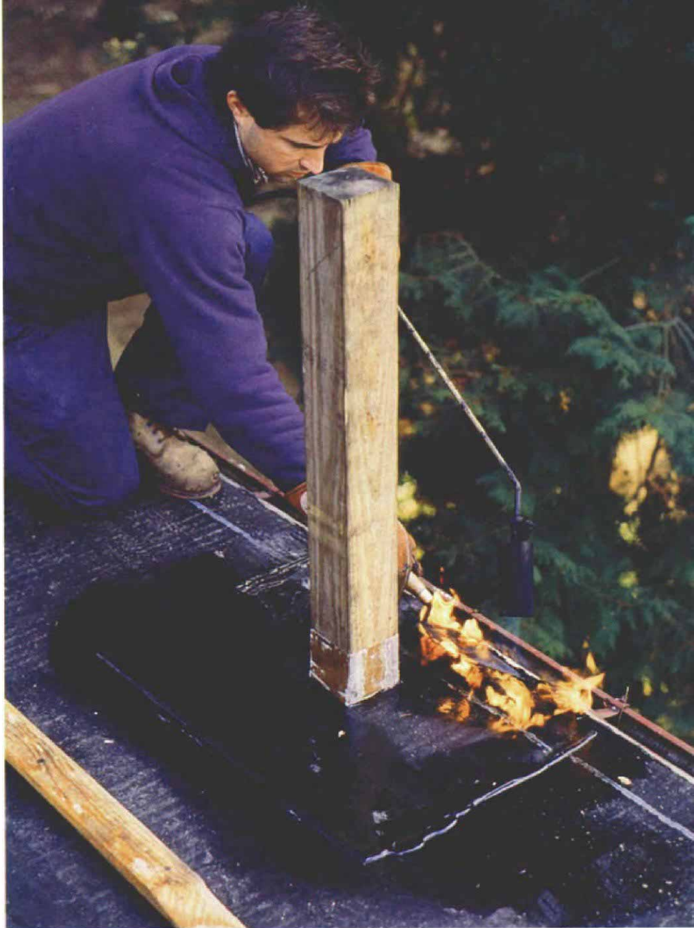
Fused flashings. One of the advantages of a single-ply modified-bitumen roof is that repairs and alterations can be heat-welded to the membrane long after the initial installation. Here, flashing strips of bitumen, which cover the copper base flashings around the 4x4 posts, are being fused to the roof membrane.
