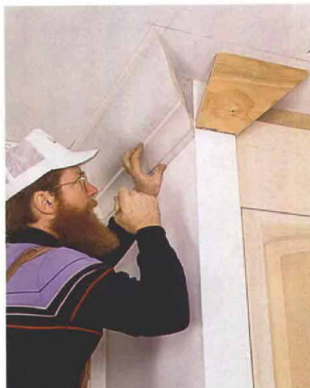
Test fit. After affixing the top portion of the crown to its backing blocks, Mosher checks the fit of its corresponding bottom half.
