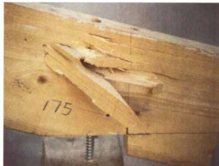
Overloaded lag-screw connection.
