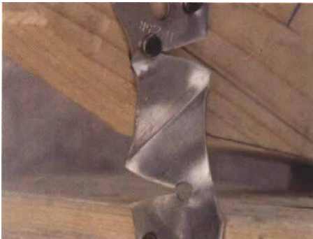
Overloaded rafter-tie connection.
