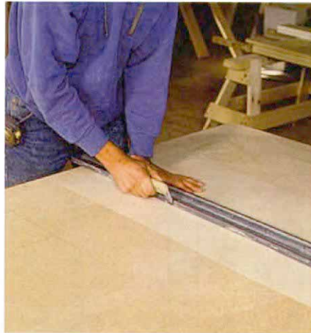
Low-tech, but effective. To cut laminate with a scoring tool, draw the tool across the laminate several times. Then, holding down one side, lift up on the other, and the laminate will snap cleanly along the score.
