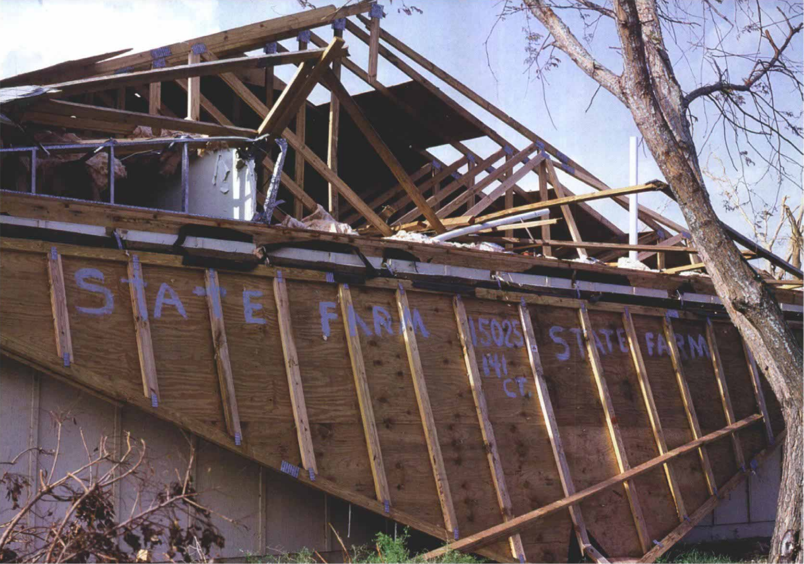
Blowout. Houses that were suddenly pressurized when a door or a window blew in often lost their roofs as the wind sought a way out of the building. With correct nailing and bracing, the roof may have survived.
