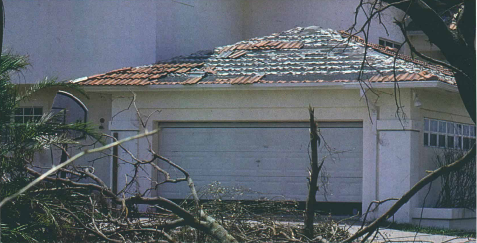
Hip roofs fared well. The low profile of hip roofs helped them deflect the storm better than gable roofs did. But tiles didn't always hang on the way they should have. The horizontal lines of mortar under these tiles reveal an incorrect installation.
