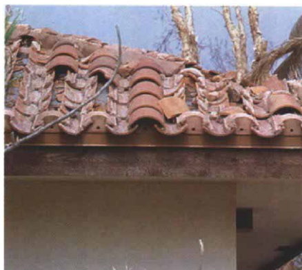
Two-piece barrel tiles. The leading edges of some cap tiles were snapped off by the wind, but the trough tiles remained.
