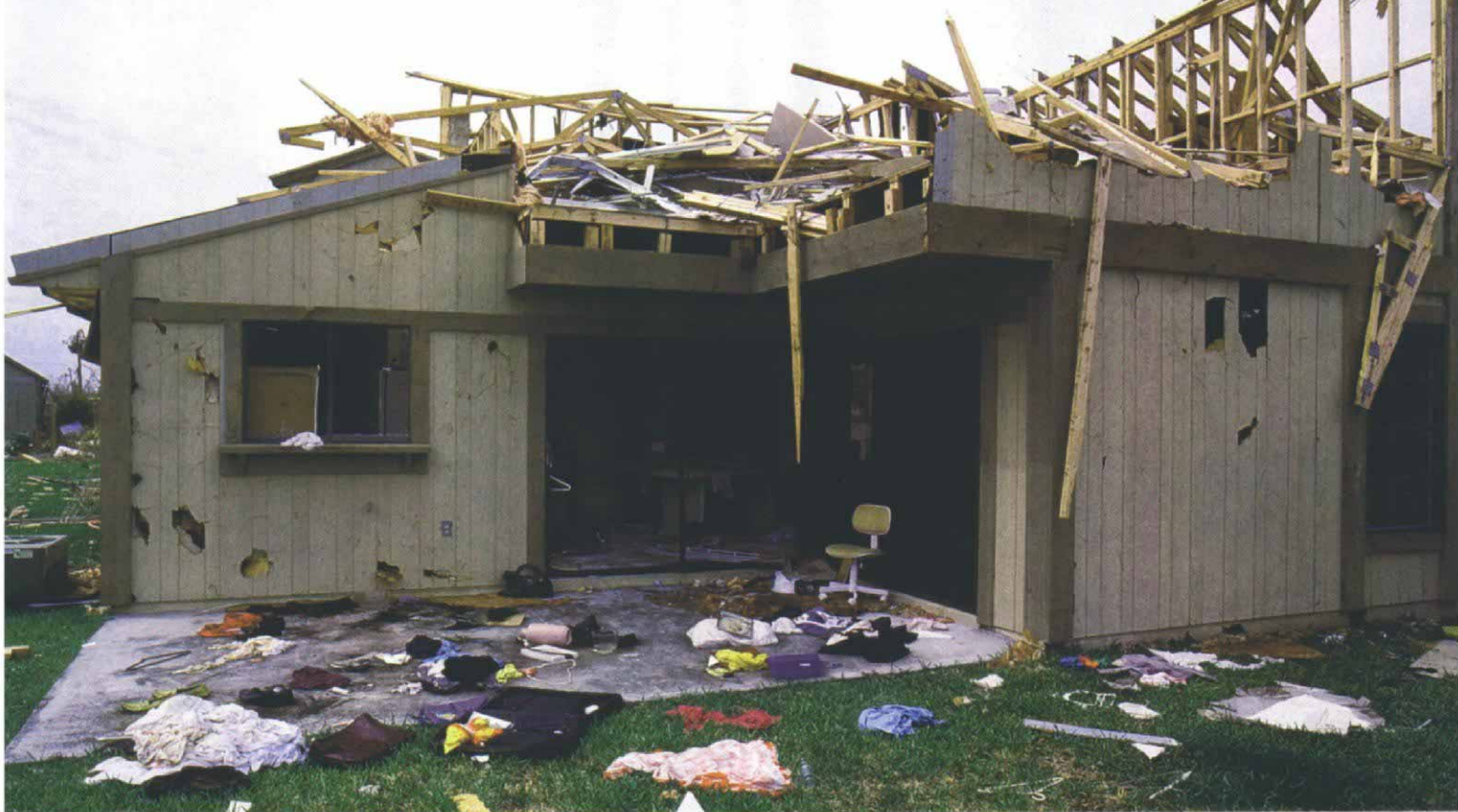
Hardboard was no protection. Wood-framed walls covered with 5/8-in. exterior-grade gypsum board and hardboard siding were easily penetrated by flying debris.
