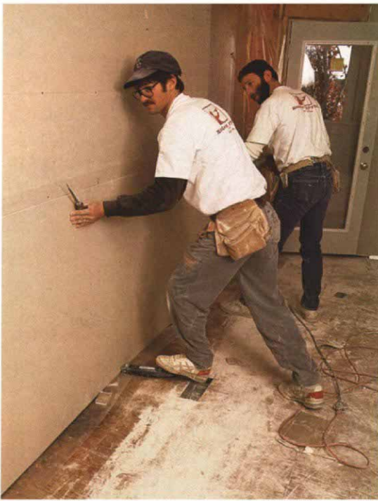
It sure beats a pry bar. A panel lever slides easily under the bottom of the sheet and wedges it into place.
