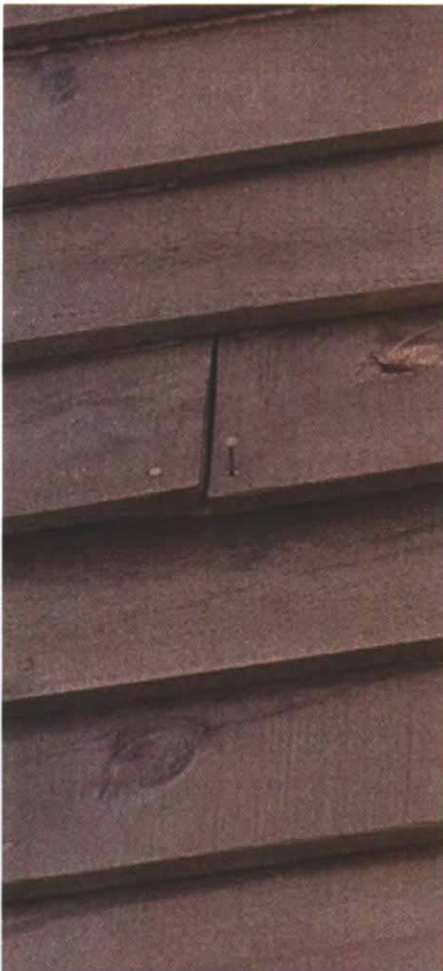
Nail pops. This siding has cupped, pulling out the nails. Back-priming the siding and using longer nails would have helped.
