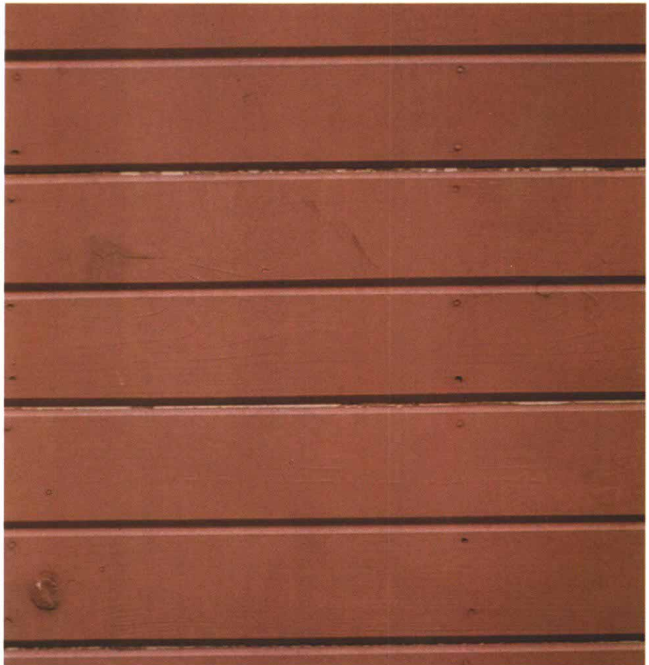
Exterior siding shrinks. This T&G wood siding dried out after it was painted, exposing unpainted surfaces between some of the boards. The problem would have been avoided had the wood been allowed to acclimate on site before installation.
