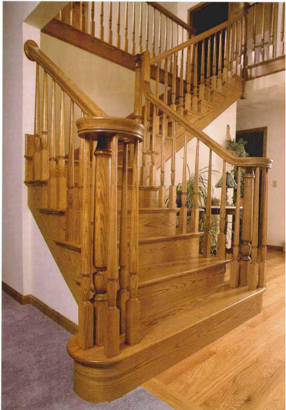
The first step. An open stair—where the finished stringers aren't boxed in by walls—makes it possible to have a double bullnose starting step. The riser is kerf-bent around forms that fit over the mitered stringers, and the tread is notched to fit in front of the second riser.
