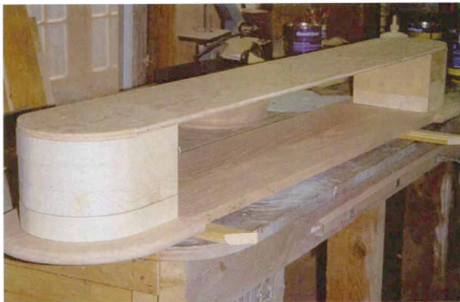
Building the bending form. By scribing around the bullnose ends of the tread with a compass, the author determines the size and shape of the bending form. Each block is made from glued-up framing lumber; the blocks are placed on the tread and are held in place with a plywood spacer.
